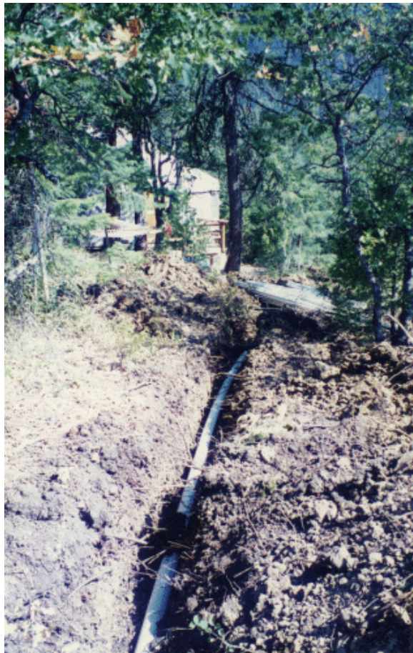
Sewer line. Flush twice, it's a long way to the Yeshe Nyingpo board meeting.
